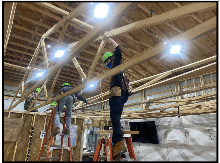
Andrew Ranger (H), Zach Ouillette (O), and Landen Caverly (H) construct the training room.
