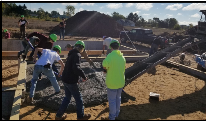
Group of Building Trades students from all four districts pouring the concrete garage floor.
