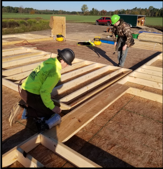
(left) Landen Caverly (H) and Addyson Hesling (H) framing the exterior walls.
